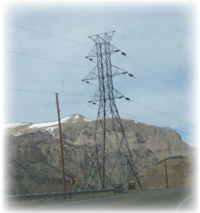
Power lines transmit electrical power generated from the waters of the Wind River.
