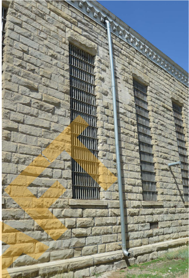
The restored wall of Cell Block A after the restoration work was completed in 2014. Photo courtesy of the Wyoming Frontier Prison.
