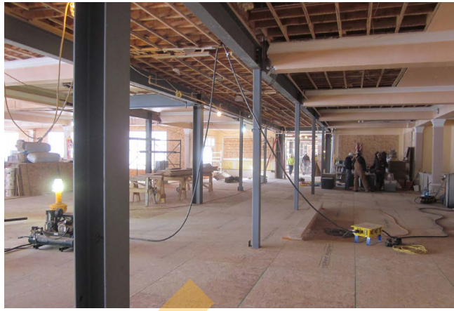
Seismic rehabilitation (2014), showing the lobby in front of the fireplace, looking towards the dining room. Photograph courtesy of Yellowstone National Park.
