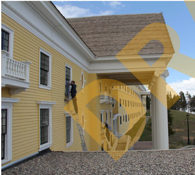
Rehabilitation project (2014). Dick Anderson carpenters installing newly restored window sash and new historically accurate window screens. Photograph courtesy of Yellowstone National Park.
