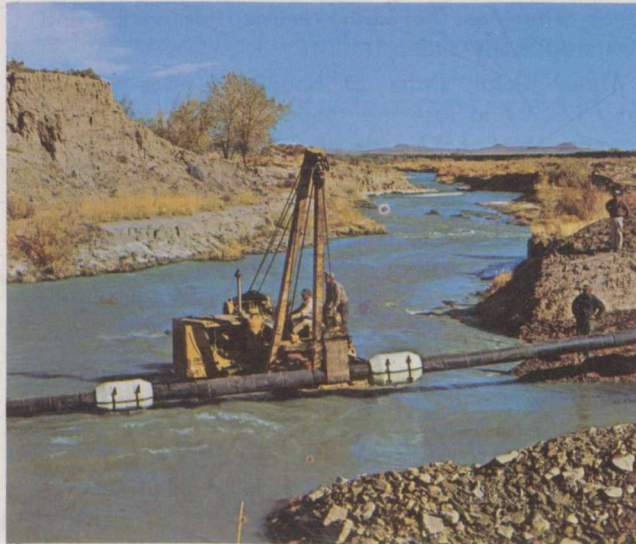
Weighted pipe is carefully lowered underwater for MDU's 10-inch Pavilion transmission line at Five-Mile Creek crossing in Wyoming. This line taps new gas sources for our interconnected system.
