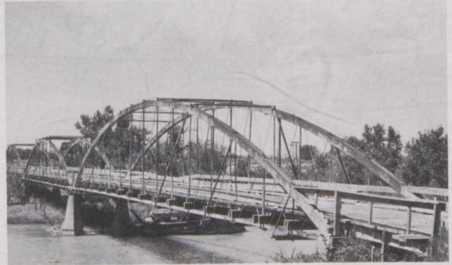
This bridge, built by the U. S. Army in 1875, spans the Platte River at Fort Laramie.
