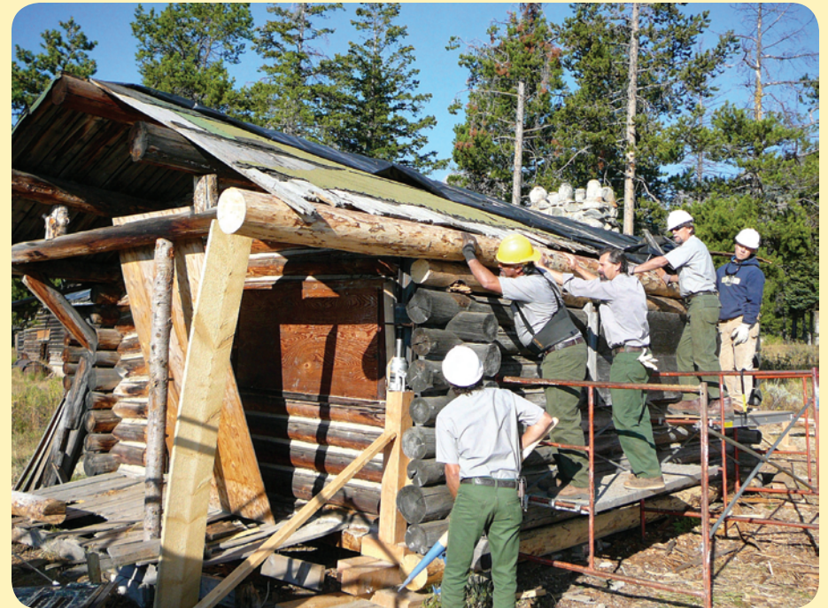
Preservation and Skills Training Program team working on stabilizing cabin 1159 at the White Grass Dude Ranch. Photo by Craig Struble.
