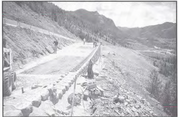
Figure 30. Installation of geogrid blocks that form retaining walls upon which the highway is built. See Figures 27 and 29 for other highway sections completed using this system. (Photograph by WDOT, Geology Program.)
