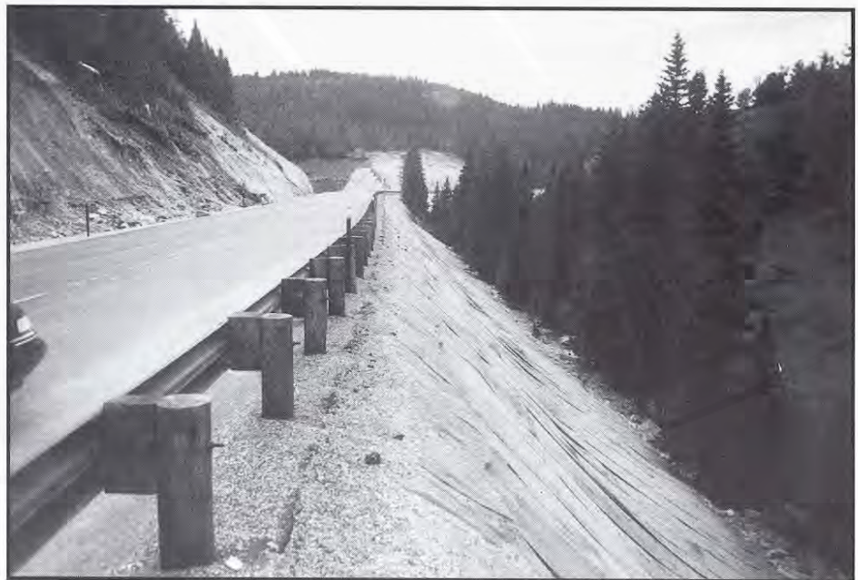
Figure 27. Geogrid reinforced fill along road through Paint Creek. View is to west. Note rockfall mesh installed on unstable backslope on left side of road. (Photograph by M.G.H., 1996.)
