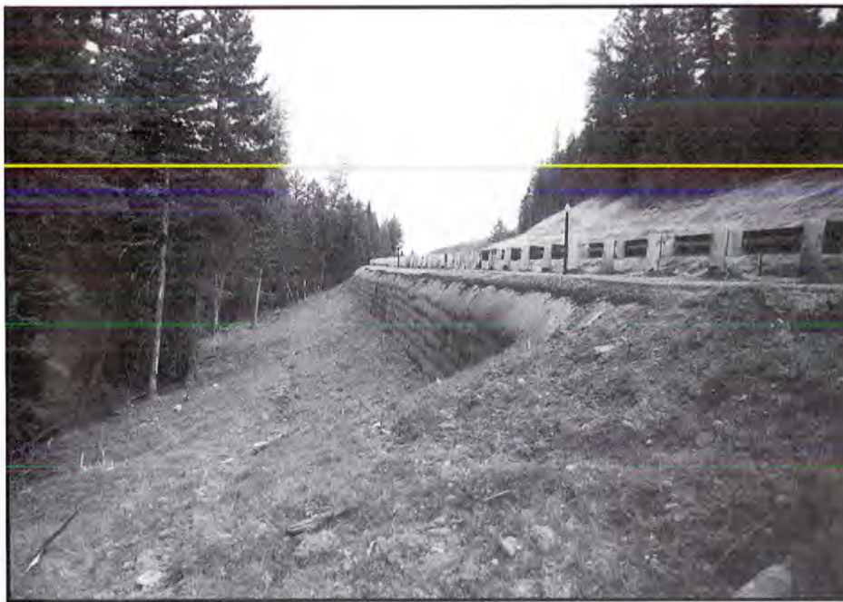
Figure 38. Rebuilt highway at Deadman Slide using geotextile wall covered with shotcrete to protect it from weather. (Photograph by M.G.H., 1992.)
