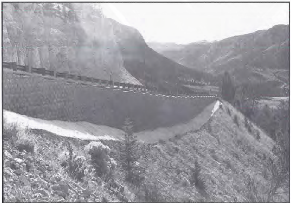
Figure 31. Completed geogrid retaining wall. Pilgrim Limestone exposed in roadcut to left. (Photograph by M.G.H., 1996.)
