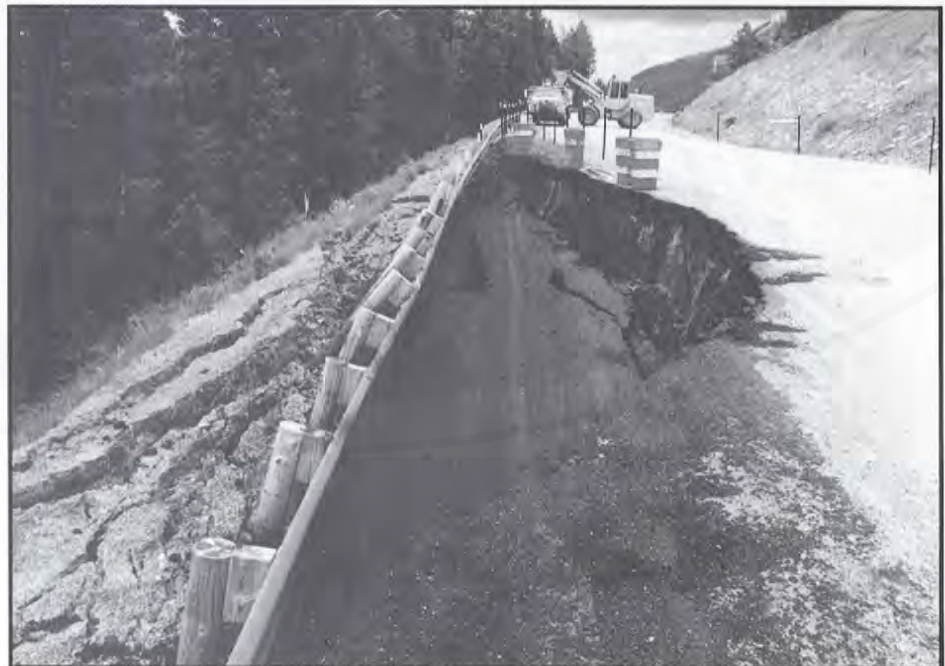
Figure 37. Highway failure caused by 1990 movement of Deadman Slide. (Photograph by M.G.H., 1990.)
