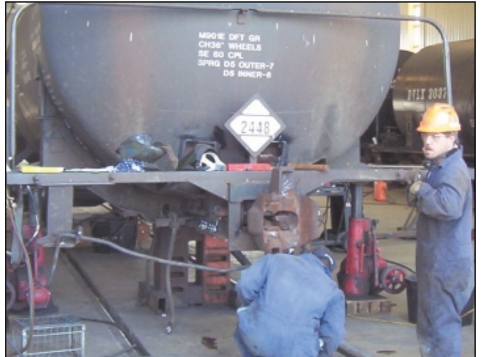
Rail-car repair specialists are working in a new facility in Shoshoni, thanks in part to more than $58,000 in start-up funding from the Wyoming Department of Workforce Services.
